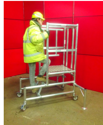
7) USE LADDER TO ACCESS PLATFORM
